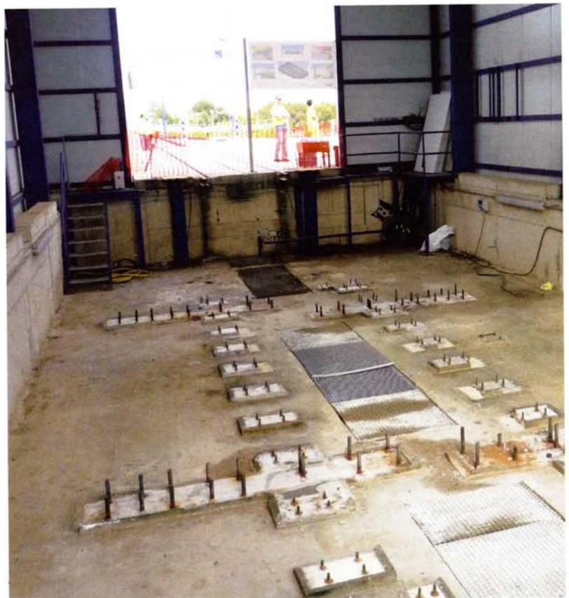
Now that one of the TCRS-1 changers has been removed from Roda de Barà, the building is being adapted ready for the installation of the TCRS-3 prototype.
