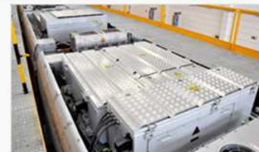
CONSUMPTION REDUCTION Of auxiliary systems
